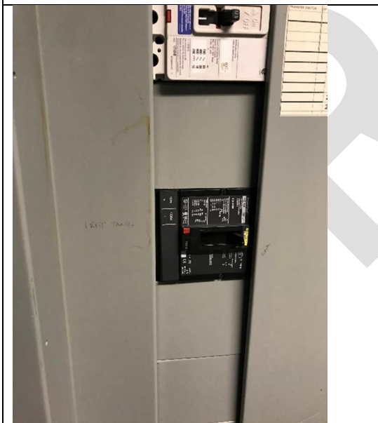
Breaker in Panel DPD for existing domestic water heater
