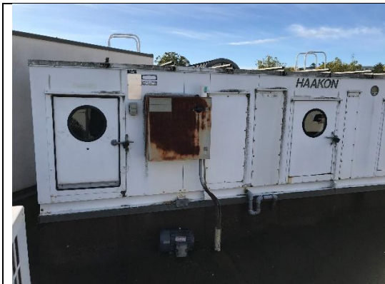
Existing disconnect for AHU-1 DX cooling coil
